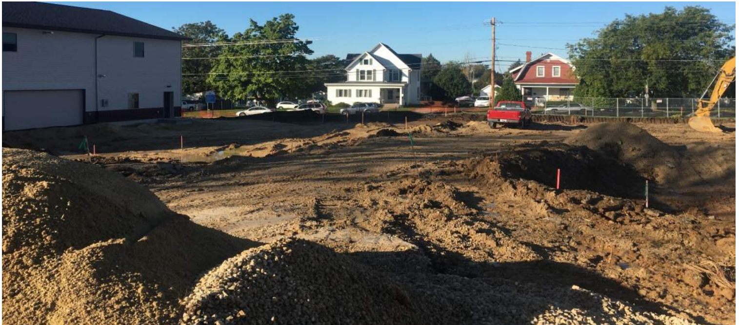
The old rehab lot is now being taken out, and re-graded for a new layout that will include the parking lot, a retaining wall, and retention ponds similar to what can be seen near Oak Street.
