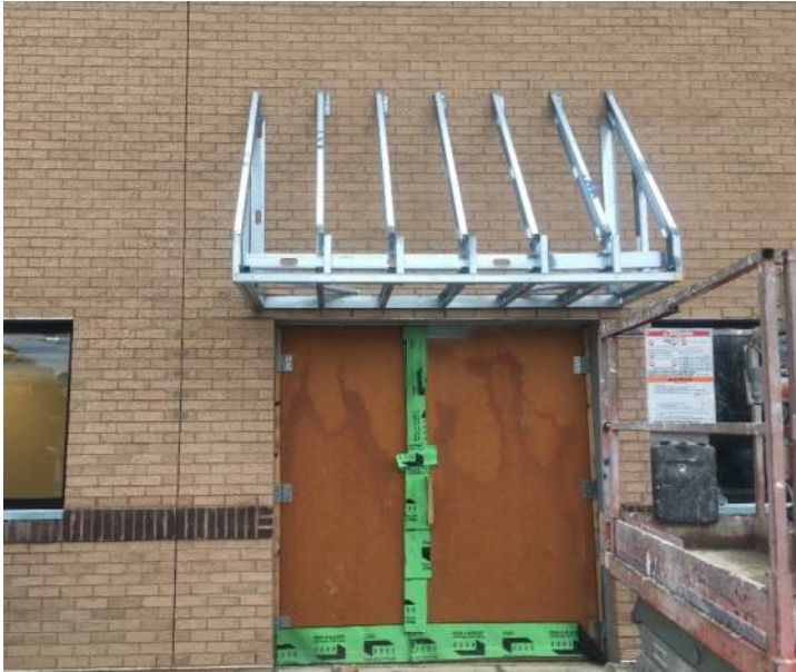
The structure for a new canopy above the Education area doors. Soon the temporary doors will be replaced with the permanent ones!
