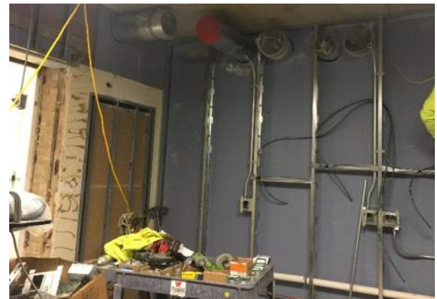
Walls and mechanical work being put into place in the new Pharmacy area.
