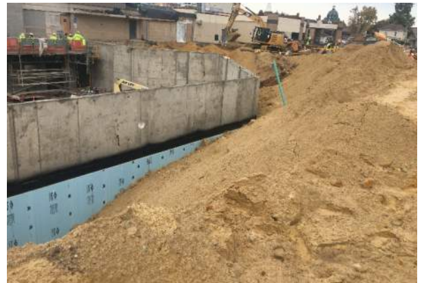
Backfilling around the existing structure for the new Clinic / Med Surge area seen to the left.
