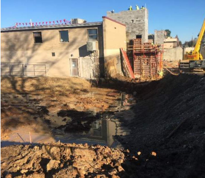
A view that captures some of the new construction, as well as the excavation where the old Rehab lot and retaining wall sat.
