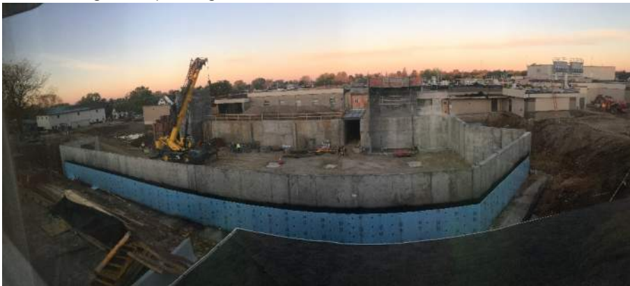
The field workers getting right to work after sunrise in the new Clinic / Med Surge addition area.
