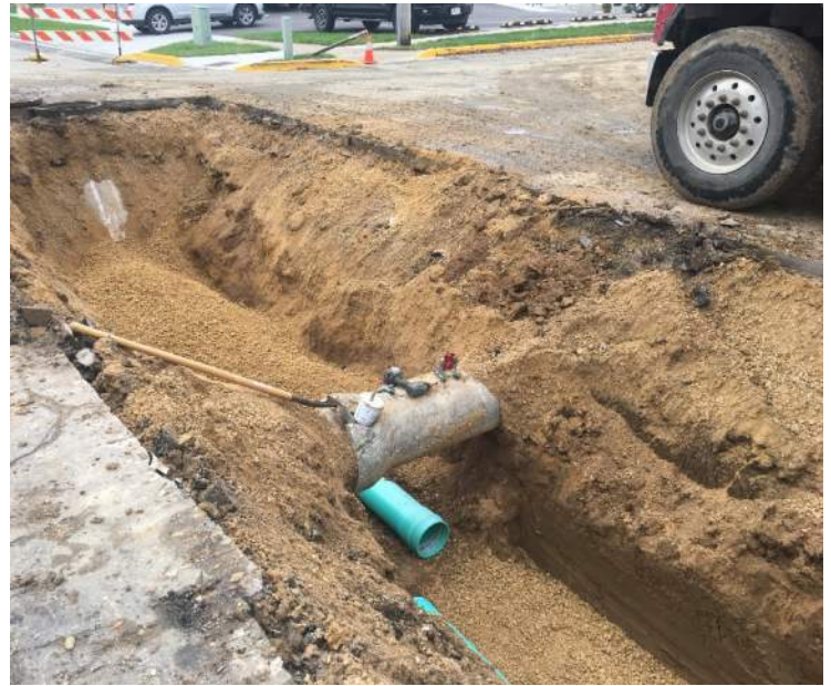
Utility work is being performed near the corner of Lincoln and Monroe Street. These new utilities will lead to the new addition at GRHC.
