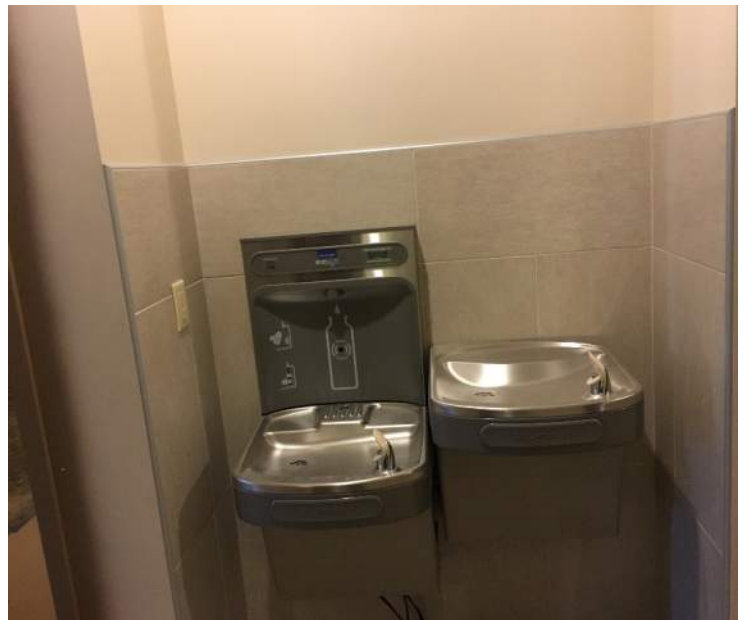
A new water bottle filler / drinking fountain combination station located in the hallway of the new Education area.
